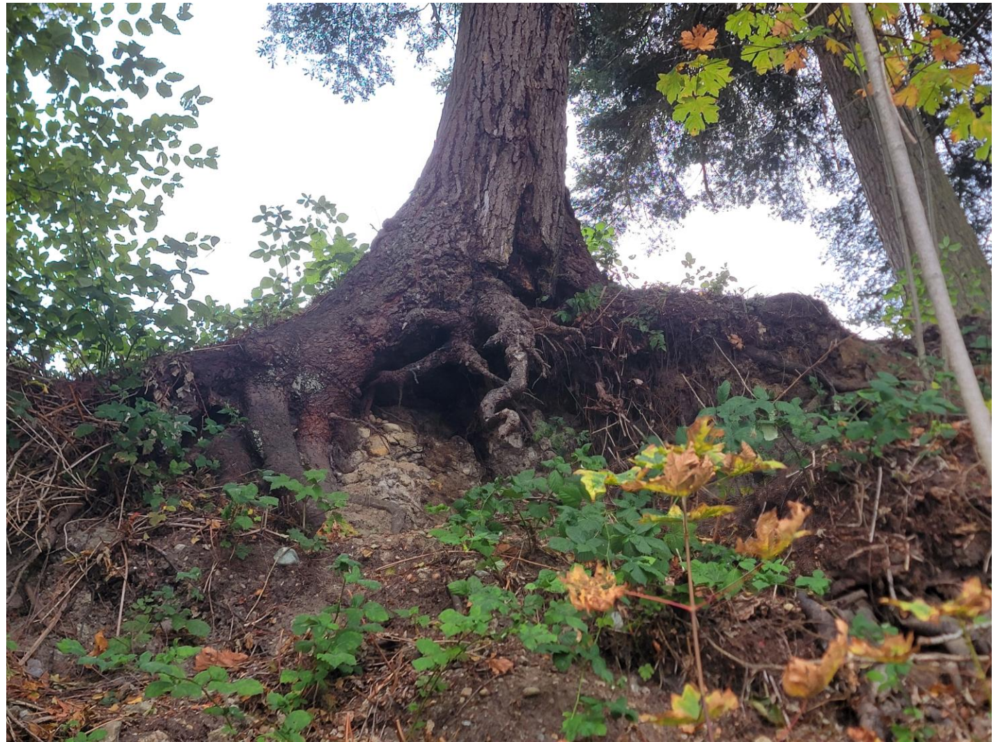
Developed area - failure bad for septic. Still good for the beach. 3-ft deep cavity under tree.
